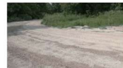
Mixed road surfaces
