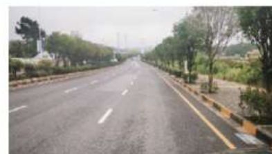
Mixed road surfaces
