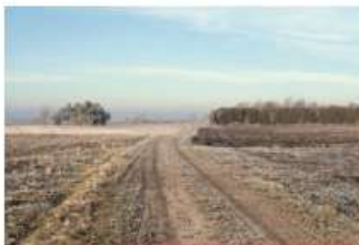
Poor unpaved road surface
