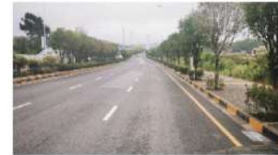
Mixed road surfaces
